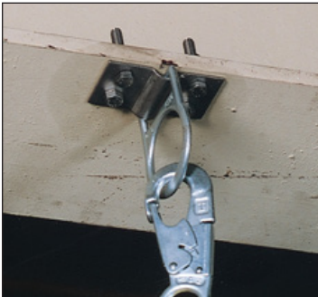
Example of a Permanent Anchor Point
